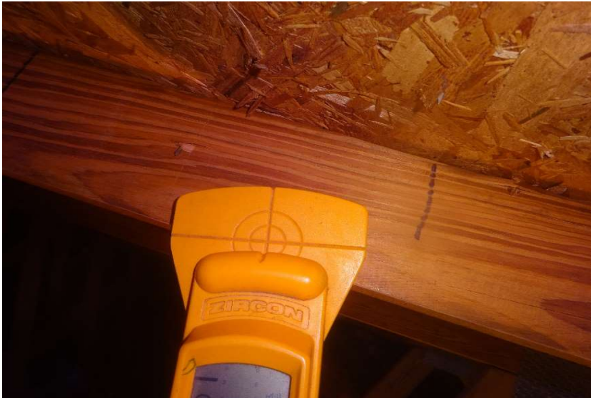
Nail location verified
